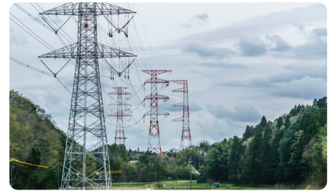
Equipment Monitoring and Data Transmission
